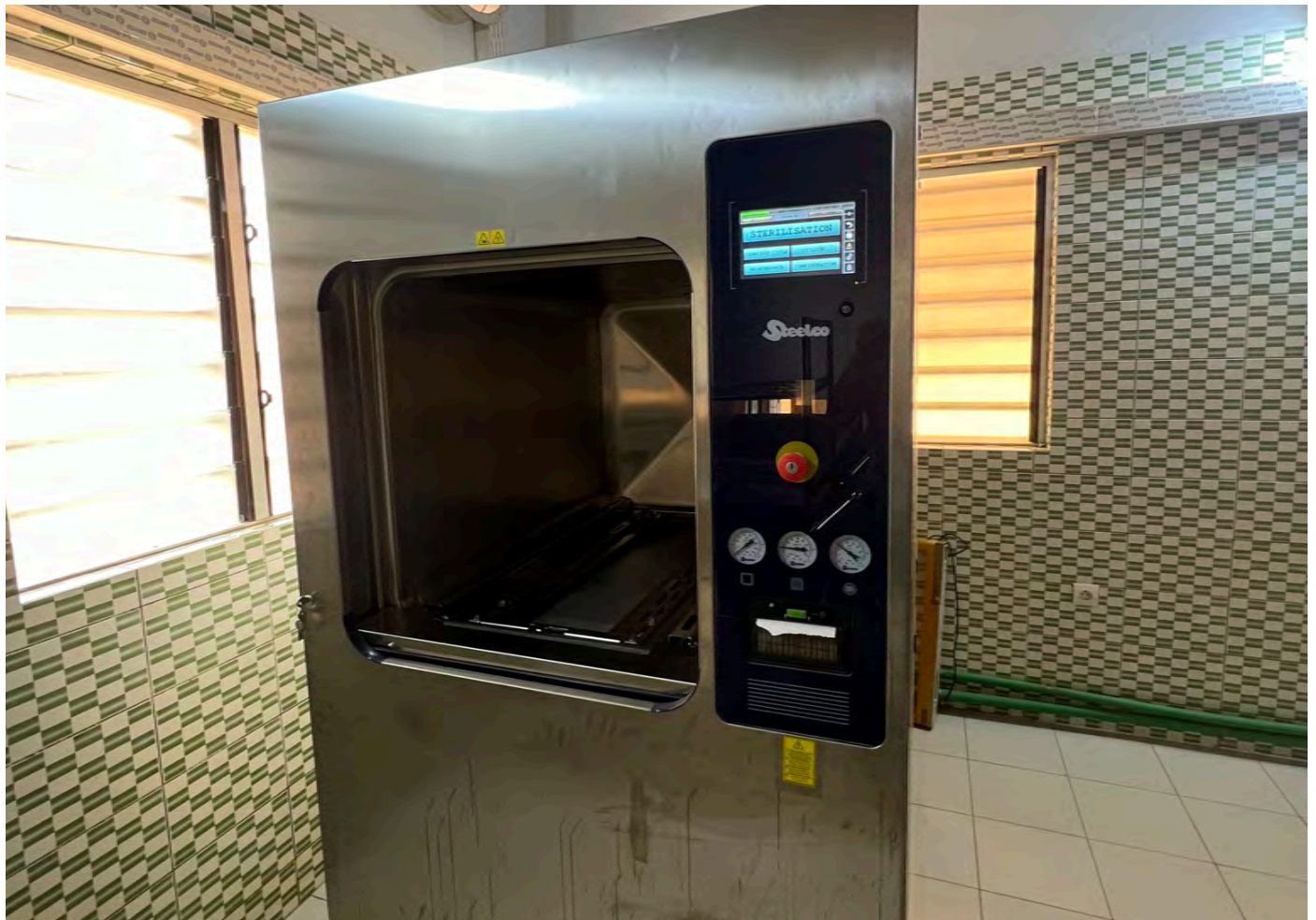
New instrument sterilisation facility
